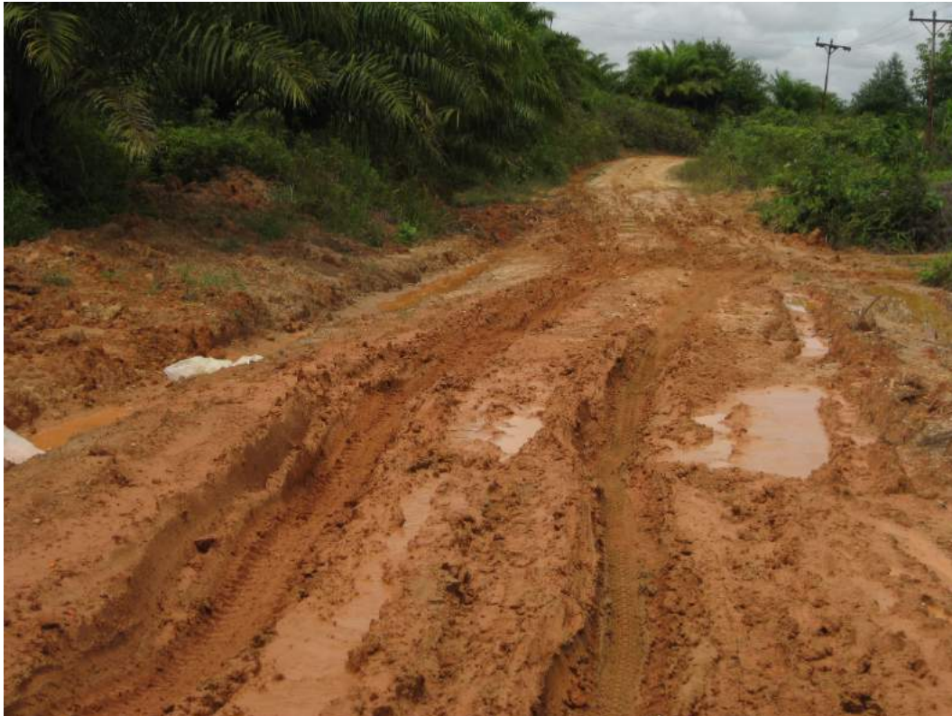
Figure 1: This road is in very poor condition and needs to be improved!
