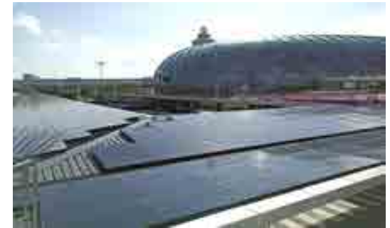
Solar panels at Changi Airport
