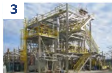
Jet Fuel & Gasoline Plant Silsbee, TX (1)
