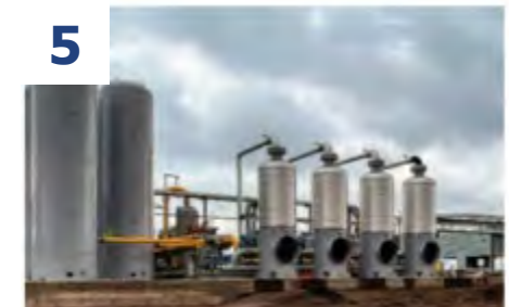
Gevo RNG Facility Operating in NW Iowa
